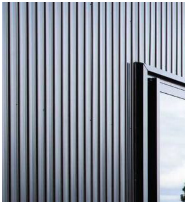
Warm grey undulated metal sheet. Clear difference between both building uses, Tenants' Hall and residential.
