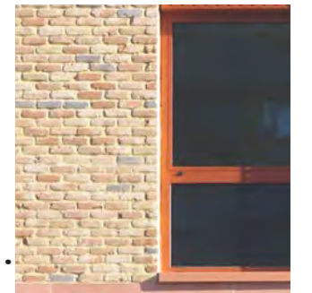
Metal frame windows - PPC finish slim frame profile - opaque fritted glazing to lower panel
