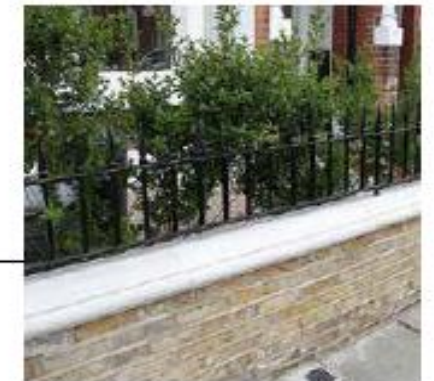
Low brickwall with railing on top. Brickwall to be made with protrusion to ensure no flat topping for people to sit and loiter.
